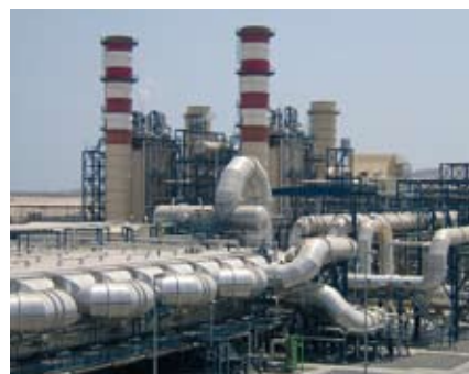
A thermal, multi-stage flash distillation (MSF) plant, in which successive condensation of evaporated brine generates energy for the next step.
