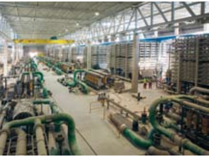
The Torrevieja 240,000 m 3 /day (63 MGD) Seawater Reverse Osmosis (SWRO) Desalination Plant located in Alicante, Spain. Designed and built by ACCIONA Agua, it consists of 16 trains of 15,000 m 3 /day capacity each with 20 PX-220 units per train.
